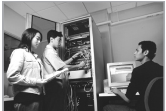
Students get to train on equipment similar to those used in industry.
